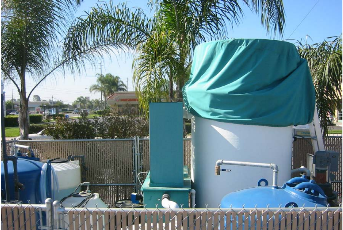
Bioreactor Operating in Stanton, California
